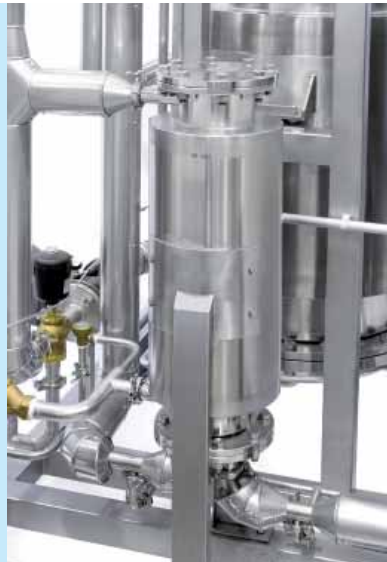
PSG 1500 T pre-heater using plant steam condensate
